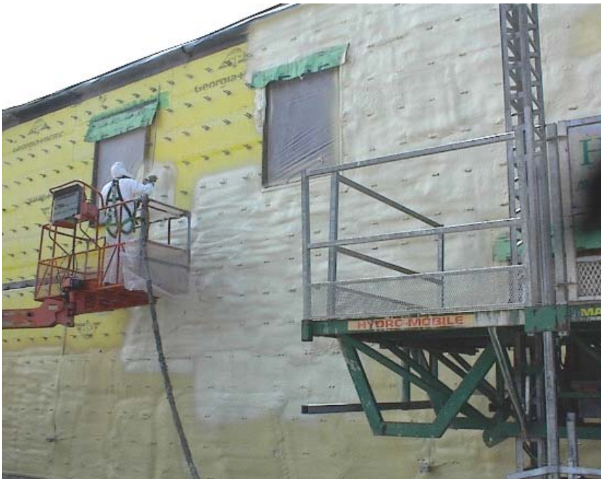
This picture shows the shell of the original building being insulated and air sealed. Construction began in 2005 and ended in 2008. The school has already seen significant energy savings.
