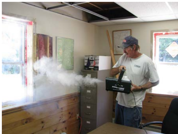
Wayne Daniels, Ingram Construction Corporation, uses a fog tester to check newly installed windows for air sealing.
